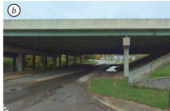
Pleasant Run Parkway North [View west] There are no sidewalks or protective curbs to serve Fountain Square Neighborhood residents walking or cycling to nearby Shelby Street transit or bike facilities seen beyond, though space exists for both. Drainage issue is apparent.
