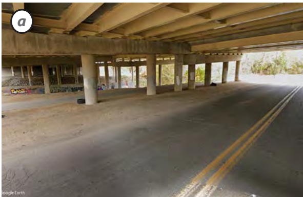
Pleasant Run Parkway South [View east] The greenway path connecting multiple neighborhoods is impacted by roadway debris and eroded exposed soils alongside an uncurbed freight and transit-serving roadway. The apparent brightness is a camera-created illusion.
