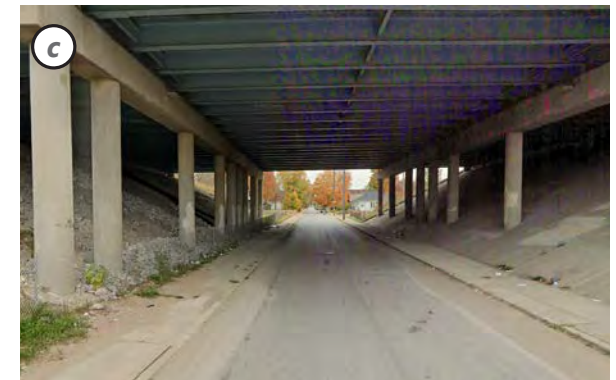
Naomi underpass [View east] Both north and south slopewall toes limit useful sidewalk width, while rubble & fencing intrudes further. The bridge drains stormwater and interstate debris towards erosive surfaces, walks and the street [not addressed by the I-65 SAFE project].
